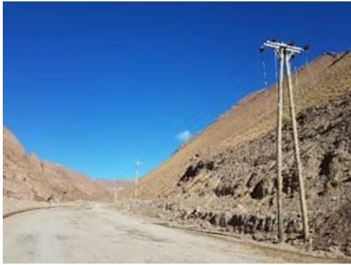
Overhead Power Line to Pit
